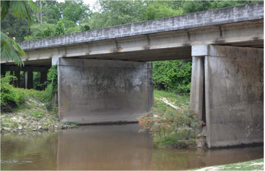
Figure 1. Typical debris deflector columns. Photo by Kathy Shelton.
